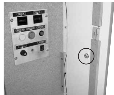
Front side of the cabinet
