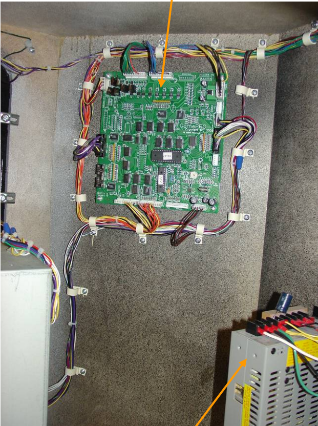
POWER SUPPLY 24VDC (5A), 12VDC (5A) CAPACITOR = NRSA222M25V PART#: UP-45 OT44-0600
